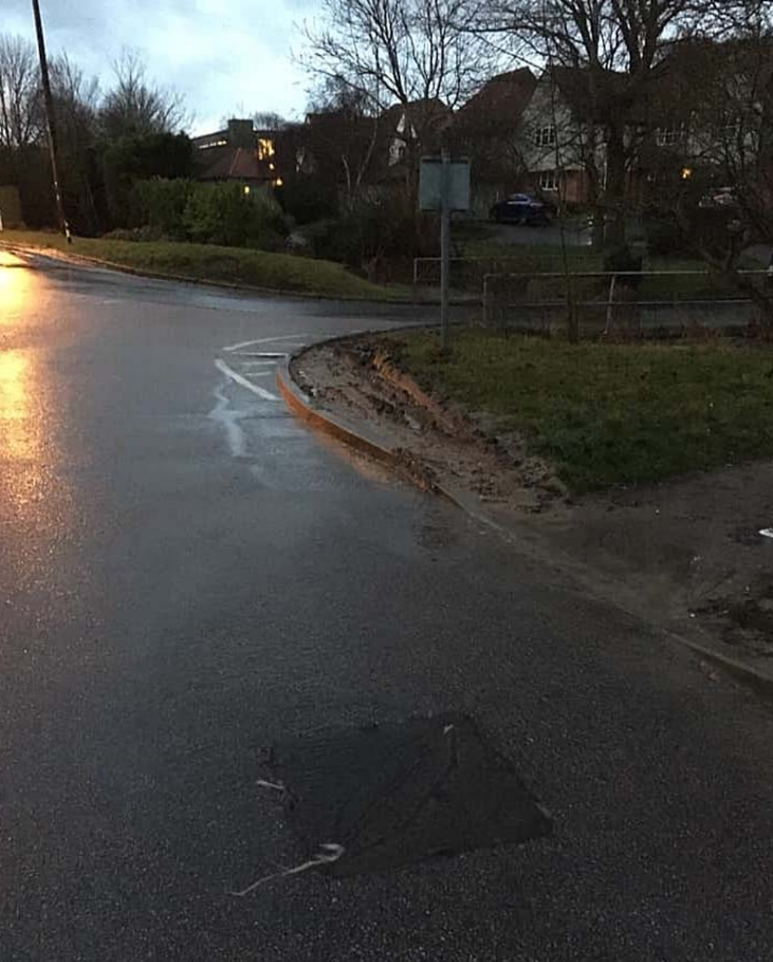
BWL 4pm 20/12/19 Drain overflowing into river
