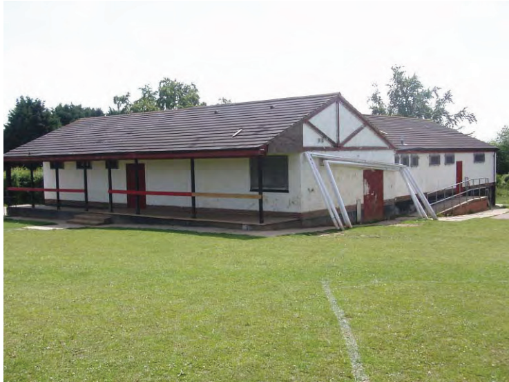
Changing facilities at Herbert Farm Playing Fields - showing signs of wear and tear
