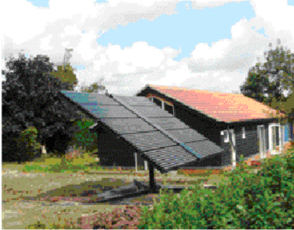
Figure 2-8: Example of a pole mounted solar water heating system that can also be used to 'track the sun' or raised above shade obstacles.
