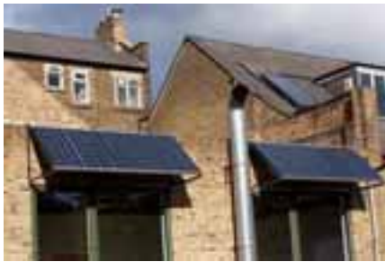
Figure 2-5: Solar collectors as canopies.
