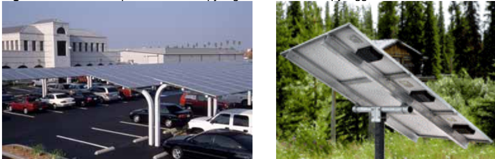
Figure 2-42: Left Example of a PV Carport Right Pole mounted PV System
