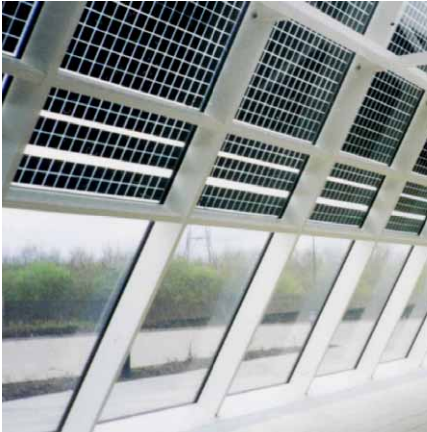
Figure 2-37: Semi-transparent PV/Glazing for PV and daylight Doxford. (Altechnica)
