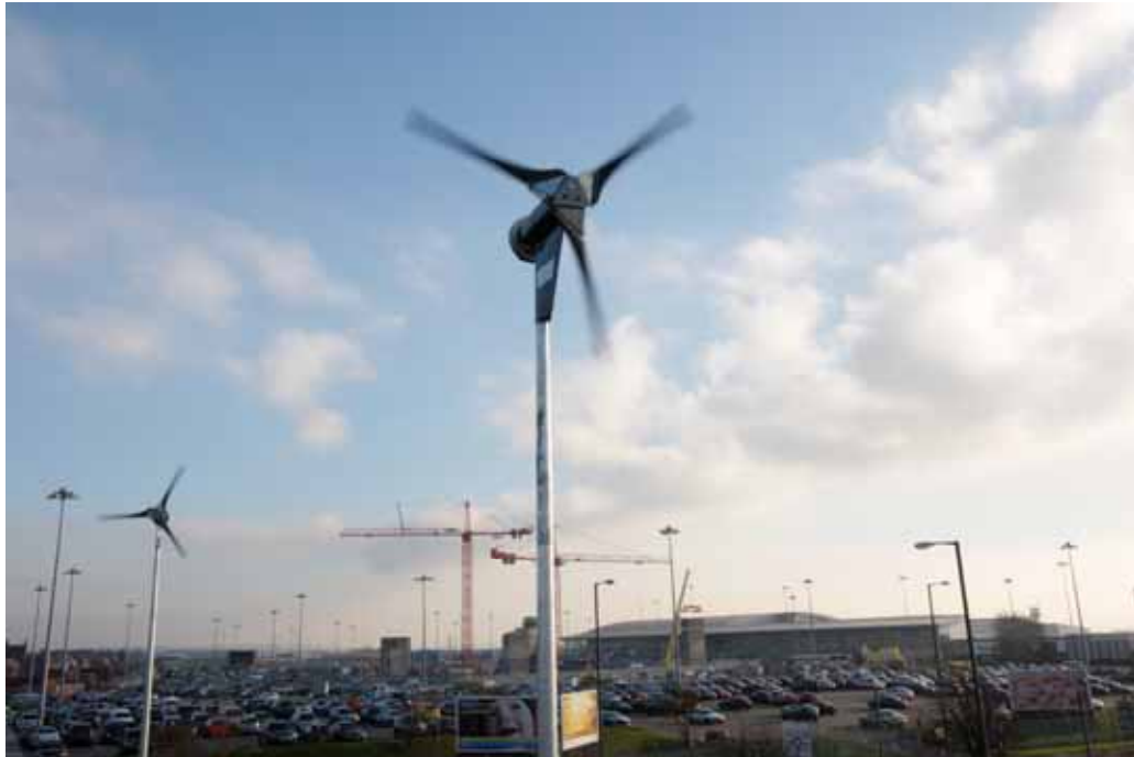
Figure 3-20: Wind turbines installed at Liverpool Airport (Source: Liverpool Airport Environment Section)
