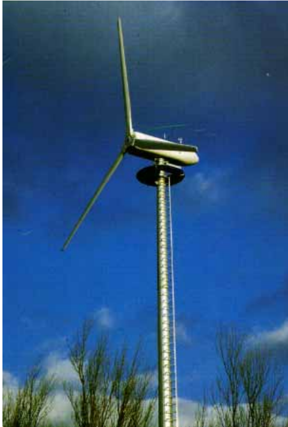
Figure 3-22: An example of a small wind turbine (20-kilowatt Gazelle wind turbine).
