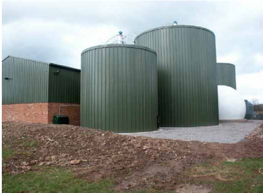
Figure 5-24: South Shropshire Biowaste Digester - food waste anaerobic digester CHP plant. Source: Greenfinch & South Shropshire District Council
