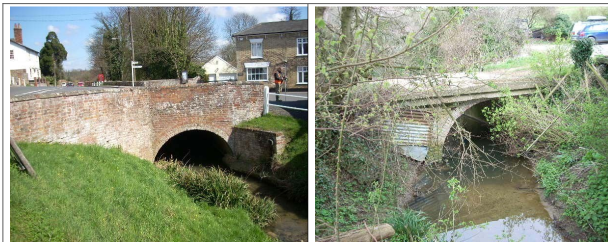
Figure 6.1 The Radwinter Road Culvert (left) and Rock Cottage access bridge (right) have the highest impacts on upstream water levels
