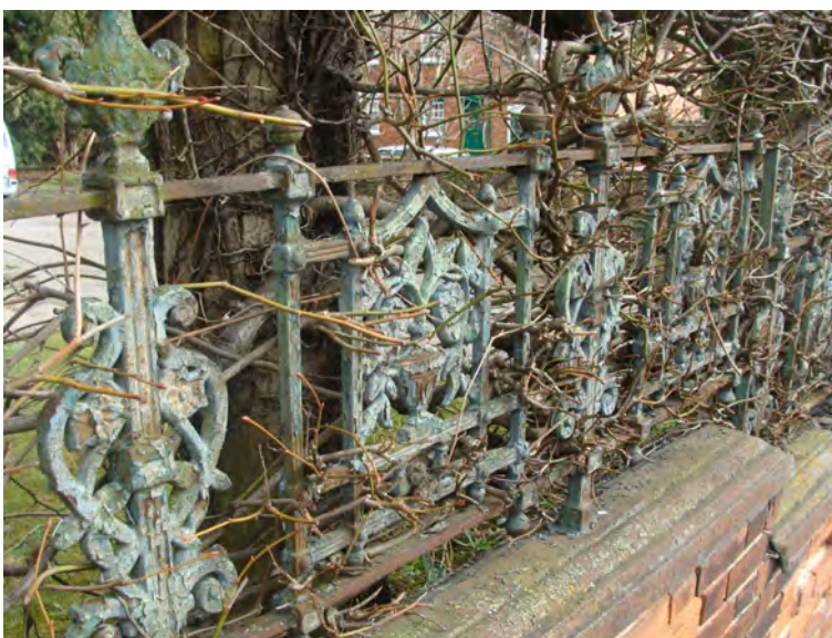
Picture 1.24 Decorative railings to Brooklyns Weaverhead lane, in need of restoration
