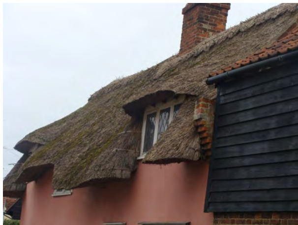
Picture 1.17 Wakelyn, a Grade II listed building with deteriorating thatch roof
