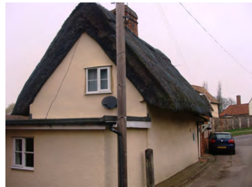
Picture 1.32 Unlisted thatched property; the thatched roof is a potential candidate for protection by Article 4 Direction
