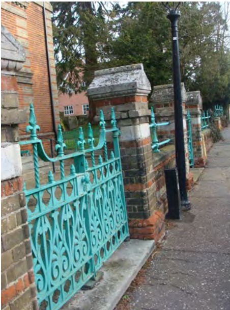
Picture 1.21 Fine 19th century railings to front of United Reform Church in need of repair
