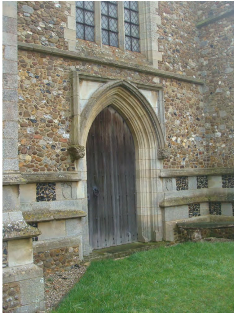
Picture 1.11 Detail of lower part of church tower rebuilt in 1882. The rebuilt tower differs in detail to the original
