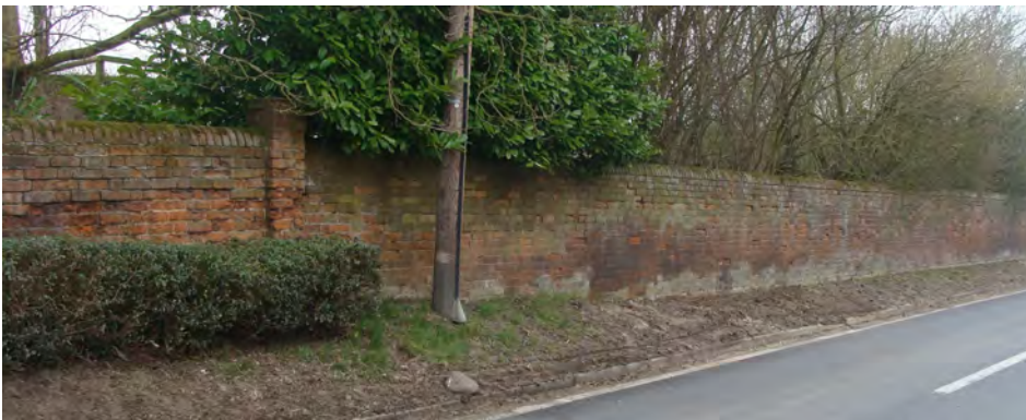
Picture 1.14 Boundary wall to White Hall, a strong feature in the local street scene and in need of repair
