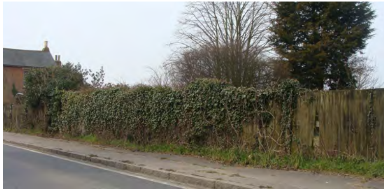
Picture 1.21 Poor quality fencing at Roding Hall paddock, boundary with B184. The ideal long term solution would be replacement with an agricultural fence or hedge of native species. The open nature of the paddock is important to the setting of the Conservation Area in this location
