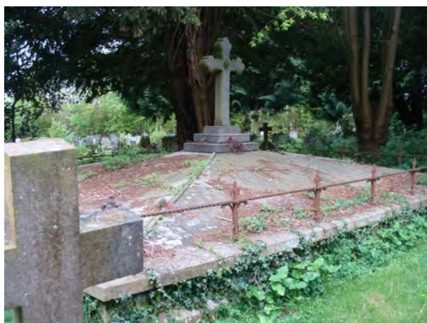
Picture 1.16 The Houblon tomb in need of minor repair and restoration. The churchwarden advised the fieldworker that contact had been made with the family in this respect
