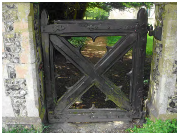
Picture 1.15 One of two fine pedestrian gates to the churchyard prior to repairs being undertaken
