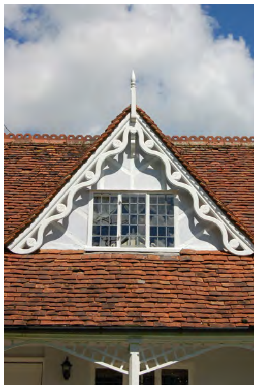
Picture 1.5 Distinctive pierced gables are a feature of many of the Maynard Estate buildings in Little Easton. These, framing the dormer windows on Church Lodge are particularly attractive.
