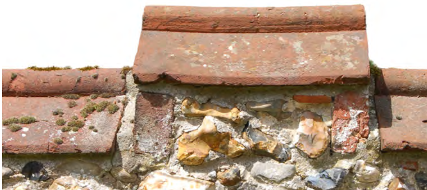
Picture 1.7 Quality brick and flint wall capped with ridge tiles at the entrance to Little Easton Manor.
