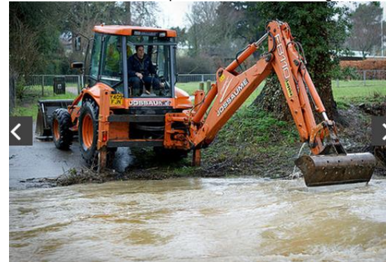
Flooding in Saffron Walden
