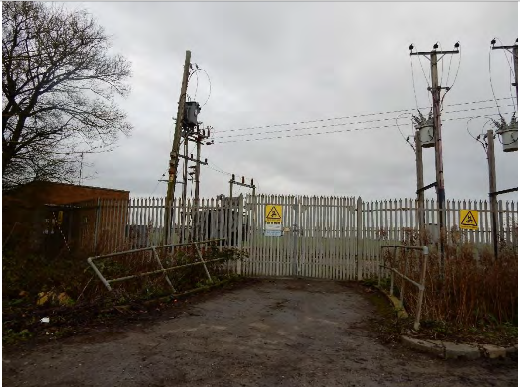
Photograph 178: View of the sub- station / sewage works in the west of the land parcel.
