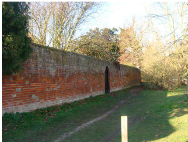
Picture 1.45 Prominent wall enclosing modern properties at Gibson Gardens. Walls both listed and unlisted are a particularly important feature in the conservation area
