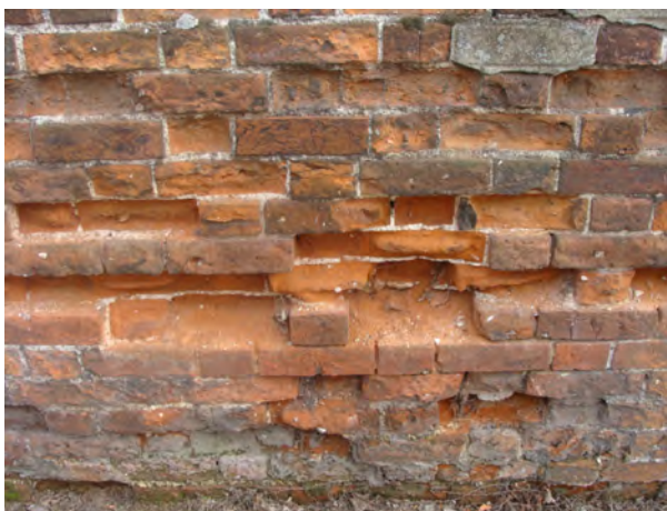
Picture 1.18 Garden wall to The Grange, Church Street, in urgent need of repair
