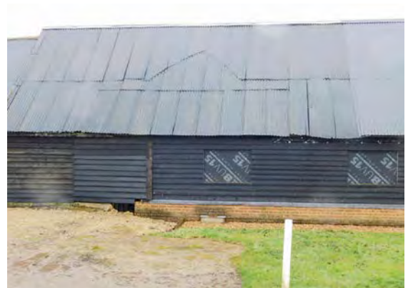
Single storey outbuilding (curtilage listed) of stained horizontal timber boarding on gault brick plinth (during refurbishment)
