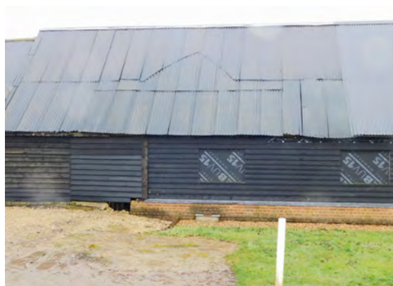
Single storey outbuilding (curtilage listed) of stained horizontal timber boarding on gault brick plinth (during refurbishment)
